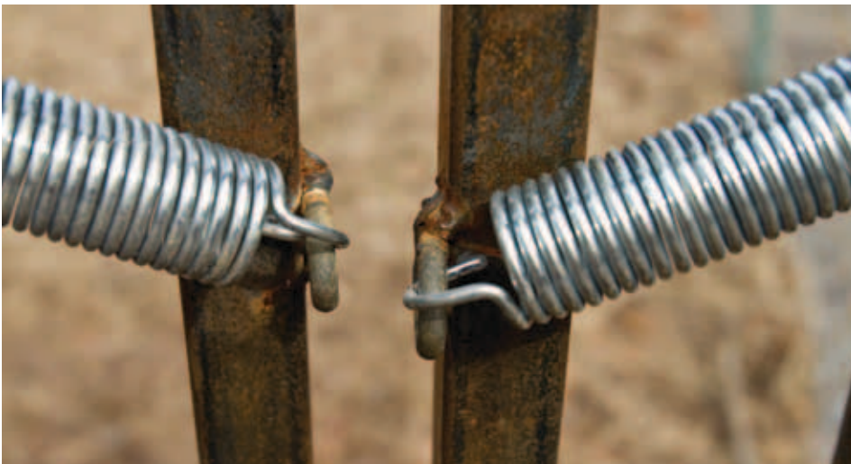
Spring door connected directly to a link of chain welded onto the door
